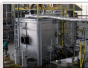
Roof burners furnace
