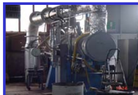
Rotary Kiln Pyrolyser
