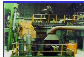
Electric Arc Furnace
