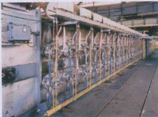
Stain less Steel Strip Reheating Furnace
